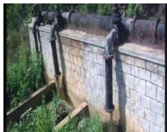
Figure 2: Sludge Drying Bed
